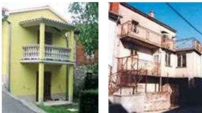
Foto 99 in 100: Neustrezne terase in balkoni v Dolu pri Hrastovljah in Padni
